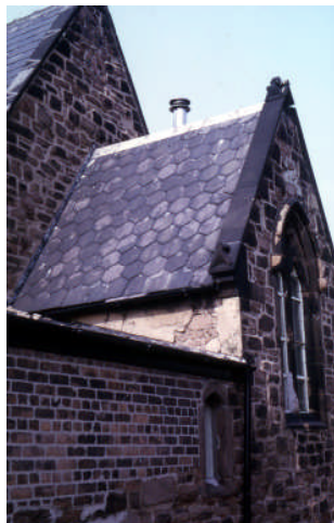
The chancel; the boys' cloakroom with interesting slate patterns. The school underwent rebuilding about 1966. Note the gas-fired flue; previously there was coke-fired central heating.
